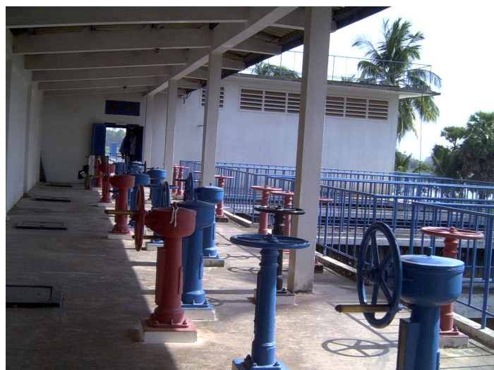
Manual Valve/Gate Operating Stands Installed in 1964
