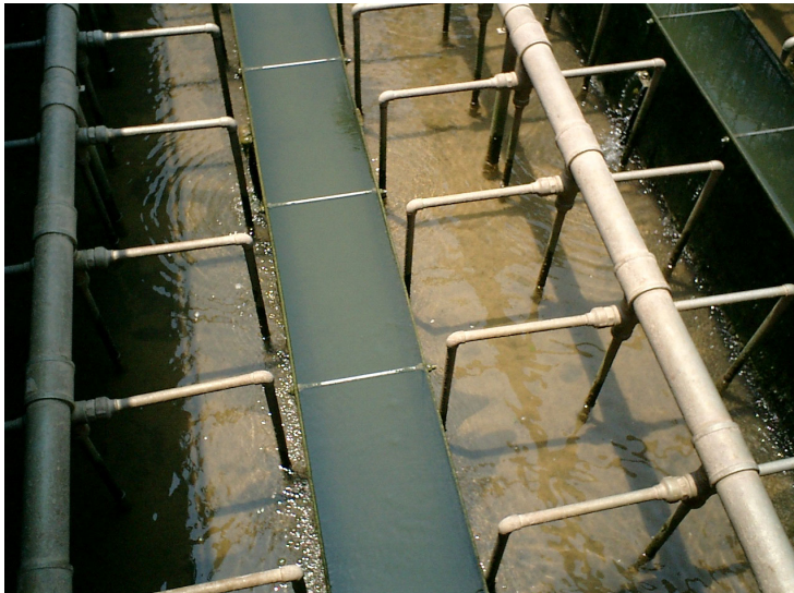
Observed Muddy Sand Bed after Filter Washing
