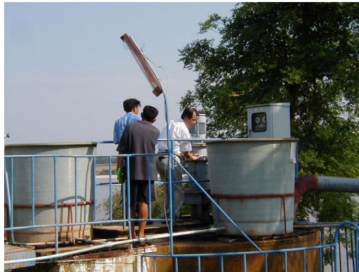
Receiving Well & Mixing Well (Polymer Feeding Tank on the Structure)
