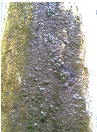
Cracks and Leakage from Cracks on Side Wall of Flocculation & Sedimentation Basin
