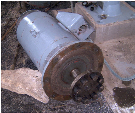
Motor of Intake Pump
