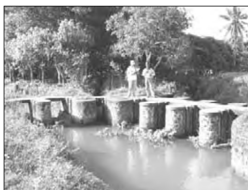
Diversion Structure, Sediments and No Control Gates
