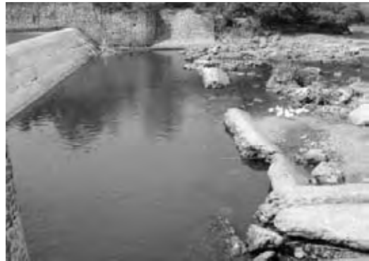
Damaged Stilling Basin and Riprap Protection
