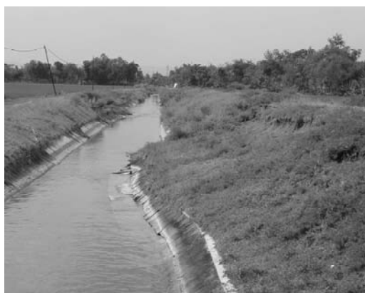
Main Canal, Sediment and Collapse at Canal Bank
