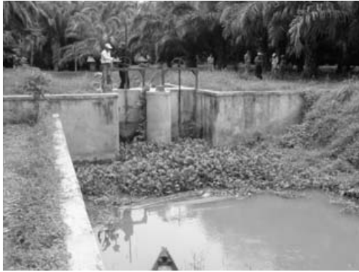
3. Condition of Intake (Free Intake System) (No O&M for a long time)
