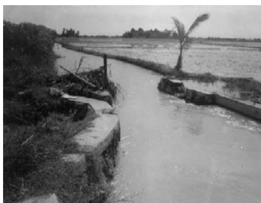
No Canal Dike and Broken Structure
