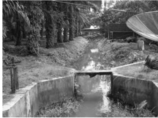
4. Condition of Main Canal at 2 km Point (Out of Services)
