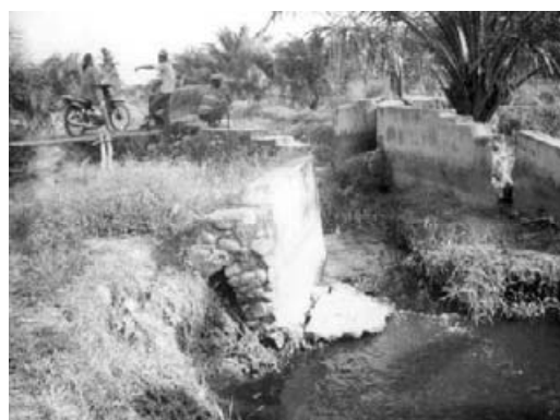
Broken Structure on Main Canal
