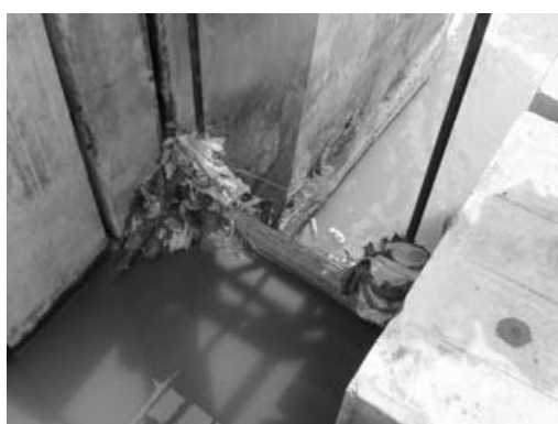
No Function of Scouring Sluice Gate
