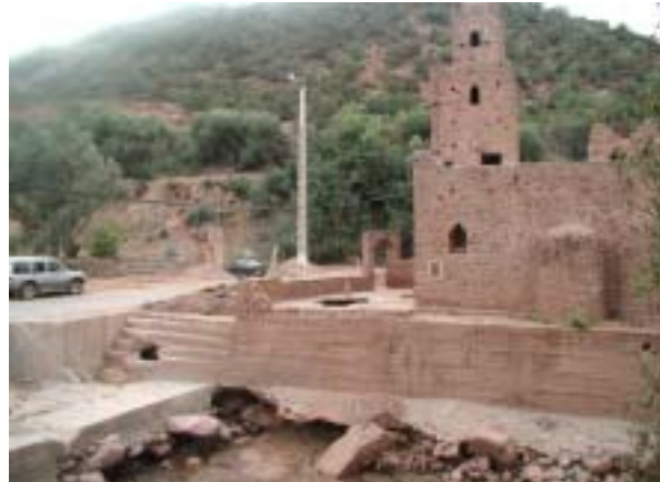
Tarzaza Tributary: The mosque was undermined by the flood water. (taken on 19 July 2003)
