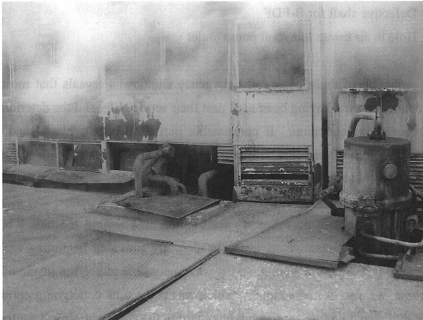
Picture 5.1-13 Steam Leaking from Turbine Area
