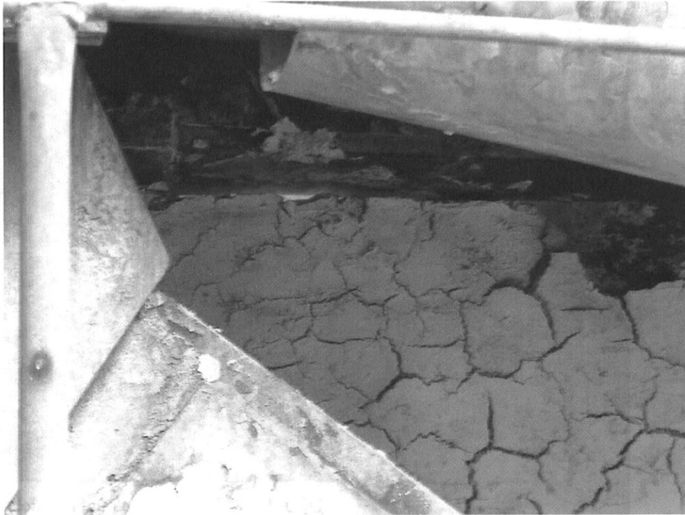
Picture 5.1-14 Cracks in Unit 6 Boiler Ceiling
