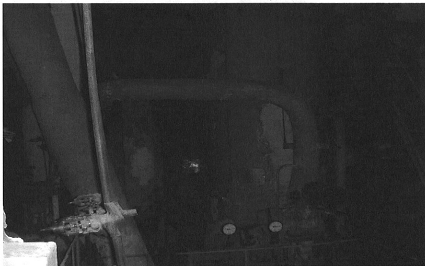
Picture 5.1-11 Inside the Turbine Auxiliaries Building
