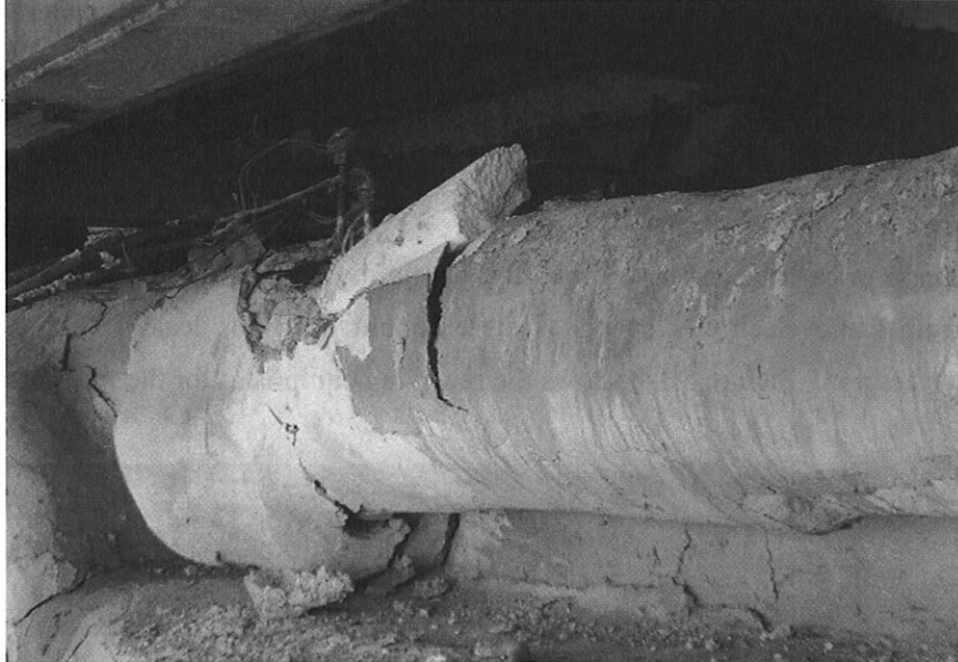
Picture 5.1-9 Pipe Missing Insulation
