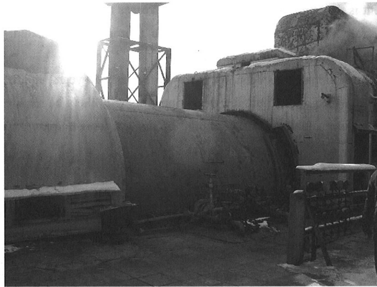
Picture 5.1-6 External Appearance of Generator
