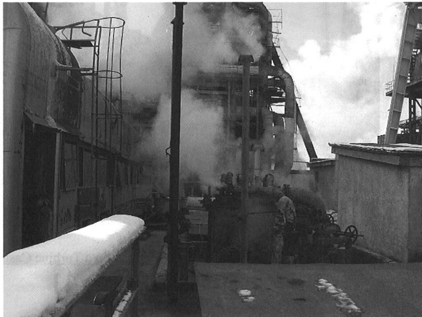
Picture 5.1-3 Condenser Vacuum Ejector
