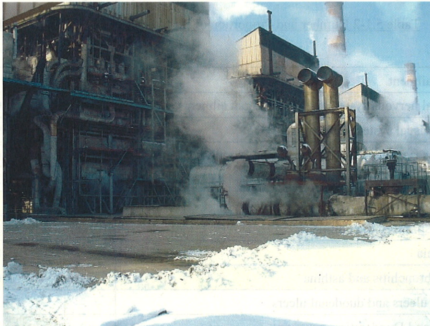
Picture 5.1-2 View of Boiler from Turbine Side
