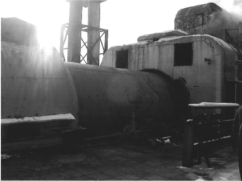
The Existing Generator
