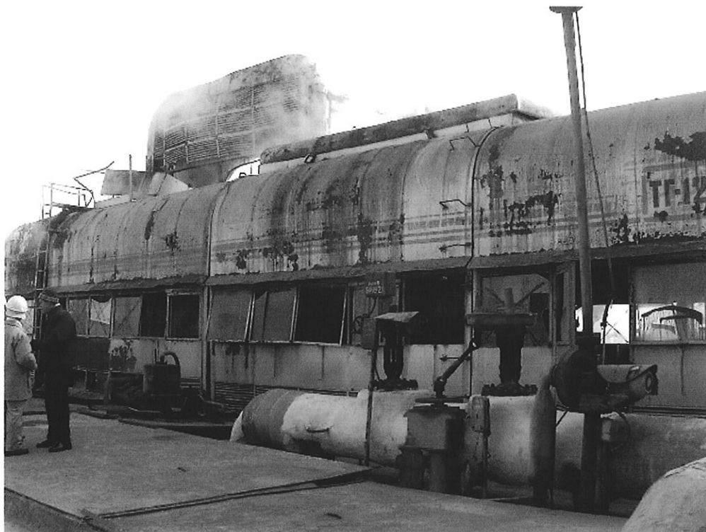
The Existing Steam Turbine
