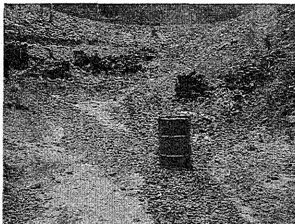
Gas Ventilation Facility (Vertical)
