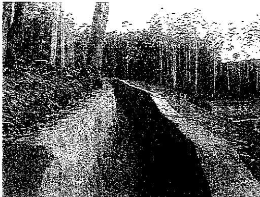
Cleaning and repairing of storm water drainage along the site (Rip rap)
