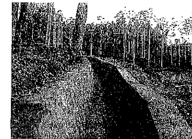
Storm water drainage
