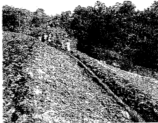
Leachate collection on the step of slope Leachate seeped to the step is collected and carried to the pond by the subsoil drain.
