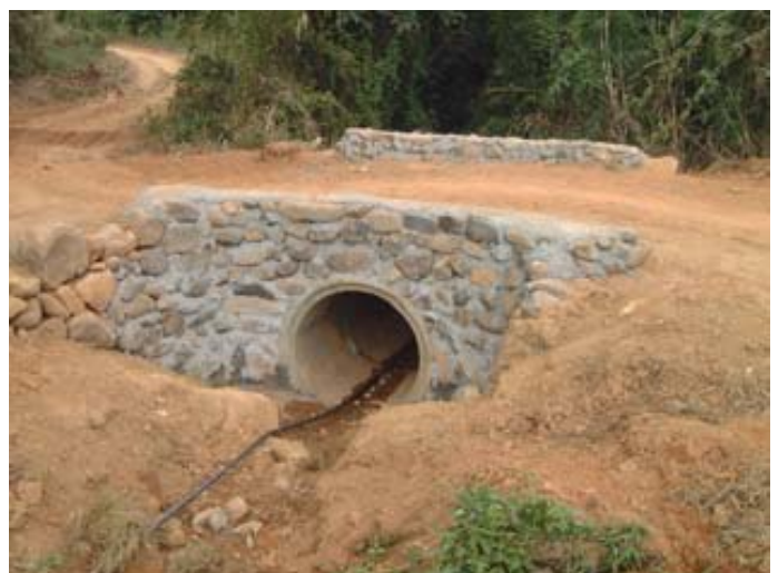
Road Rehabilitation assisted by JICA Study Team and Local Governmental Unit (LGU) (February,2003: Banila, Nueva Vizcaya Province)
