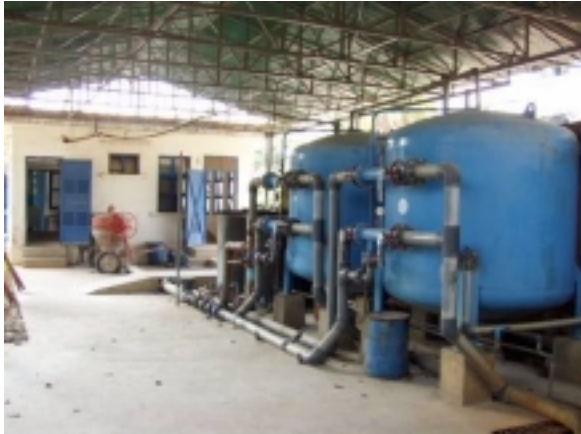
Photo 7 : Filtration units for iron removal
