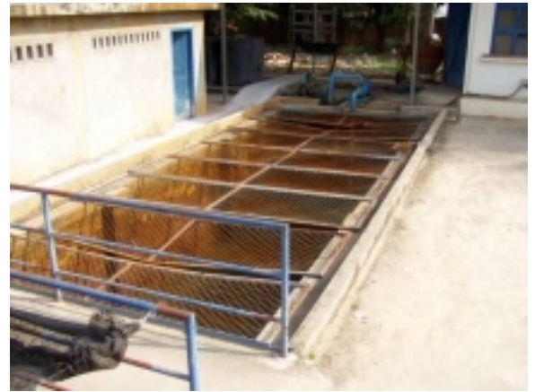
Photo 6 : Storage tank before filtration
