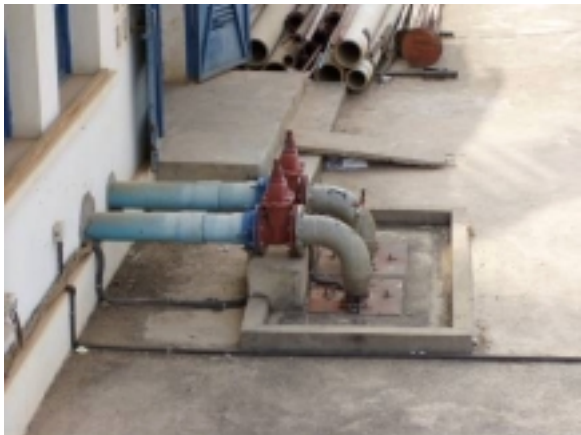
Photo 9 : Clear water lifting pumps (15 kW x 2 units)
