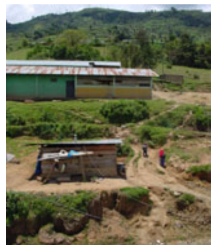
Photo2.3.7-48 The primary school damaged by the landslide
