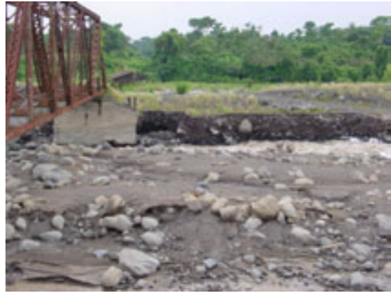
Photo 2.3.7-26 Eroded foundation of an old railroad near San Sebastián
