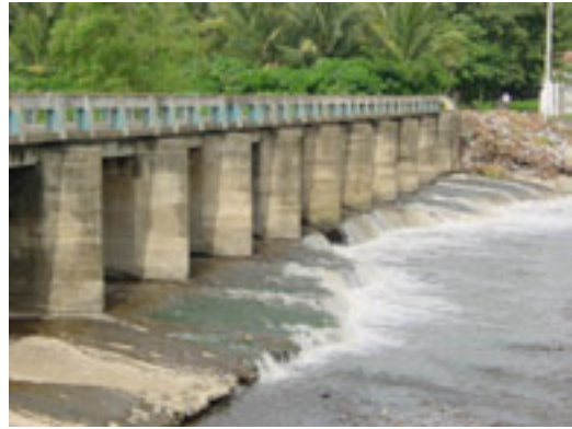
Photo2.3.7-63 Masagua bridge in danger because the foundation of bridge piers is eroded
