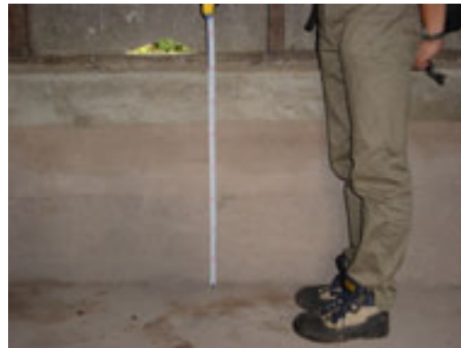
Photo 2.3.7-25 Trace of lahar on the house wall of Finca El Faro
