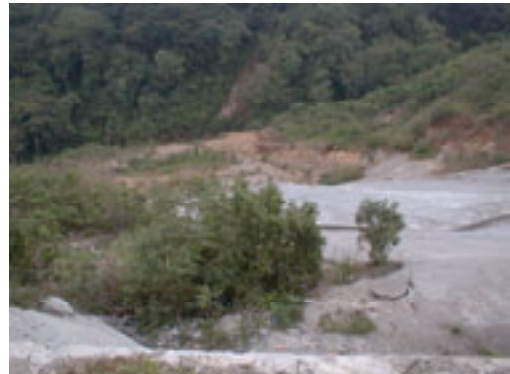
Photo 2.3.7-5 Landslide at km. 11.5 Road to El Salvador (erosion control mortar carpet were already installed )
