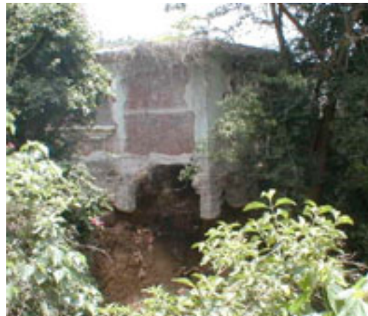
Photo 2.3.7-2 Base ground was eroded and subject to failure
