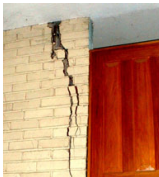
Photo 2.3.7-17 The damage of 1999 earthquake at Customs building, Puerto Barrios
