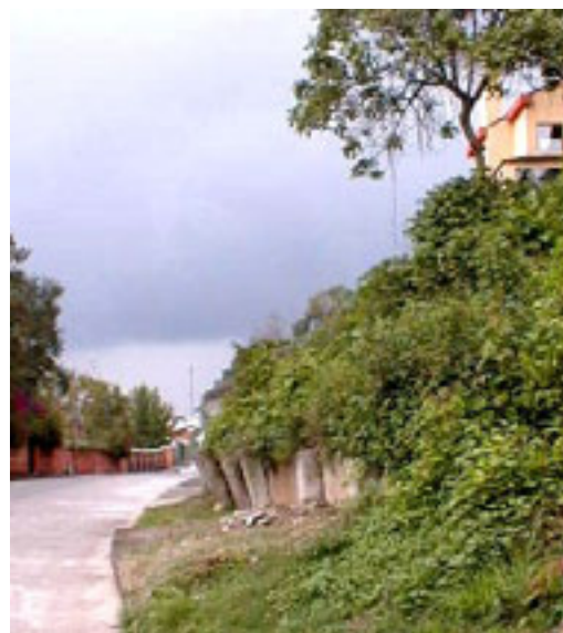
Photo 2.3.7-4 Landslide at San Rafael (the wall is sticking out )
