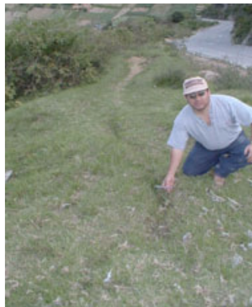
Photo 2.3.7-12 Chuicaracoj road cracking
