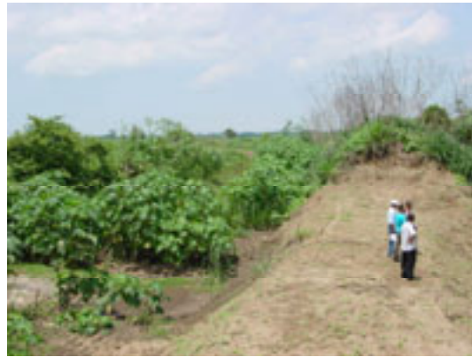
Photo 2.3.5-2 Gabions for prevention of erosion
