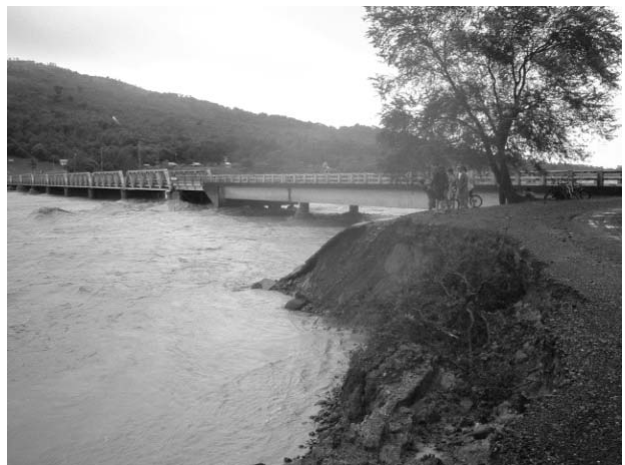
(4) Erosion of Dike at the Bucao Bridge on July 13, 2002 (Right Bank)
