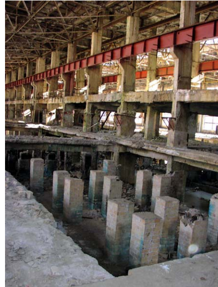
Destroyed Electrolyte Cell
