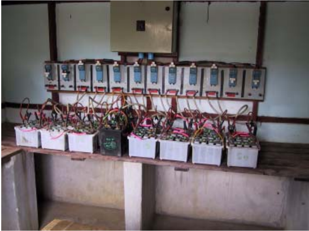
Battery Charging Station, Kone-le Village
