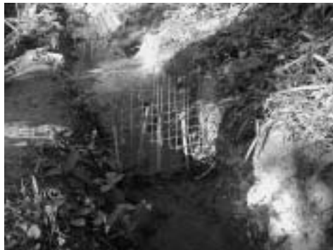
Screen on Headrace channel
