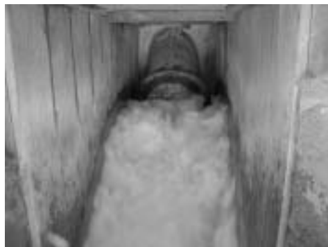
Turbine at operation
