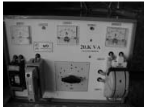
Step-up transformer 230/400 V showing rated voltage in operation
