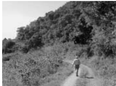
Distribution line at the longest span
