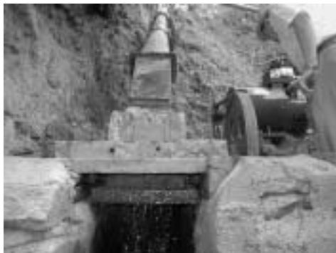
Turbine and generator
