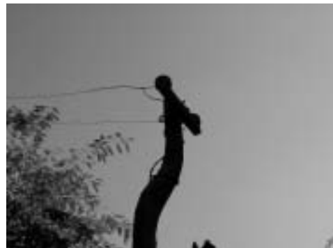
Deadend post and cable connection
