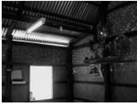
Lights in powerhouse
