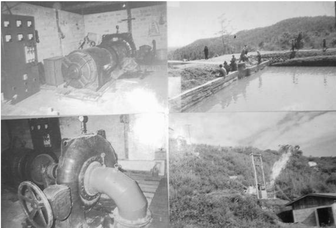
75KW Power Station for Sanpo village group, Taunggi Tsp, S. Shan State (Picture Provided by U Khun Kyaw)
