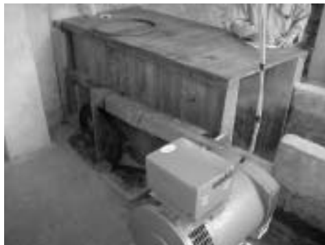
Turbine-belt cover & generator
