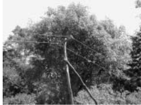
Pole and distribution line
