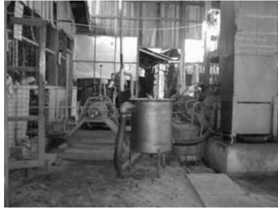
Fig.2 Tower, Filter, and Belt Connecting the Engine and Mill
