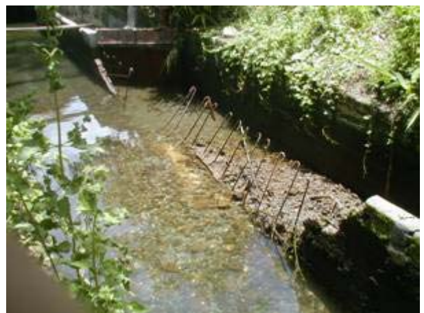
Sediments deposits in the same section.
