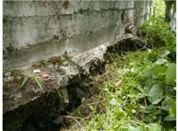
Outside foundation of leakage section (it seemed the foundation has been eroded by leakage water.)
