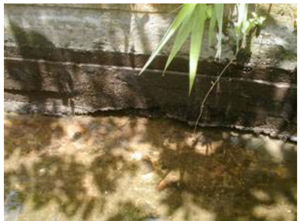
Erosion of side wall foot
