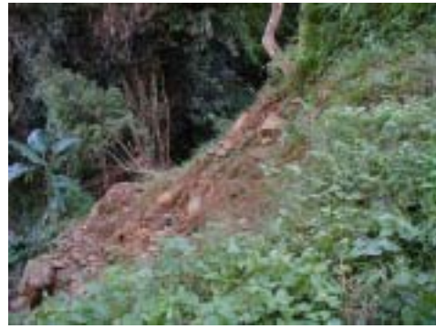
Downside slope much eroded by water
