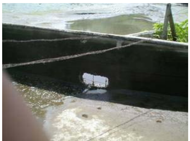
A hole is made on side wall to divert water flushing works in the Regulating Pond
