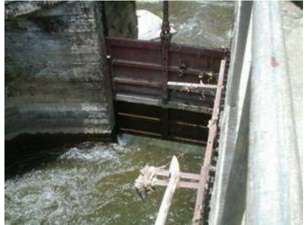
Sand flushing gate fully opened
