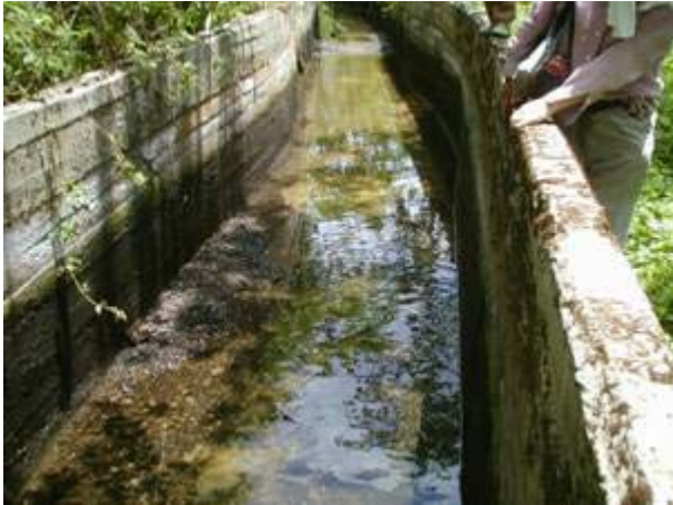
Channel floor in the leakage section right
