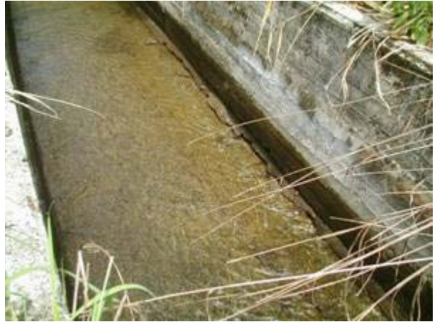
Channel floor at one of the leakage points
