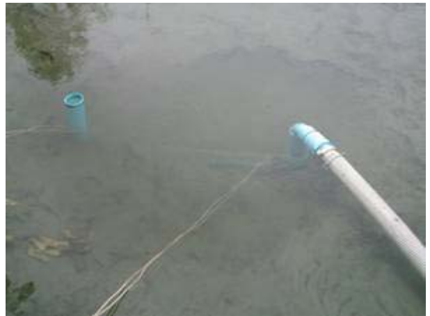
Flute under the water after sand flushing, part of horizontal pipe seen in the bottom of depression that was created by flushing sands around
