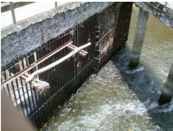
Intake trashrack and wreck of deck for operator to remove leaves etc.
