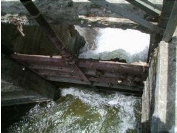
Sand flushing gate
