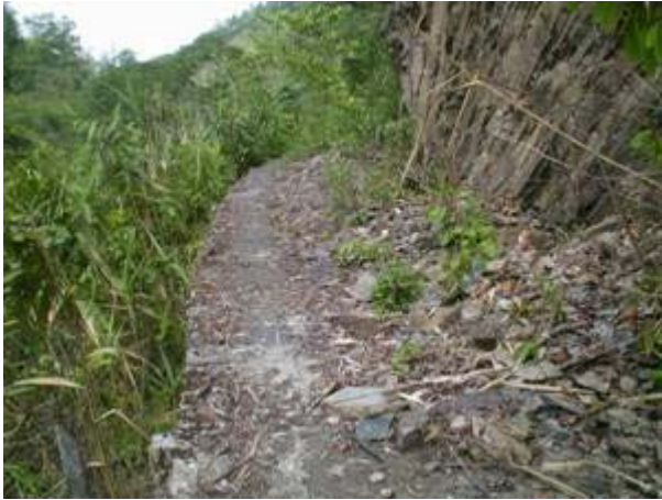
Debris on the channel cover, proving effectiveness of the cover.
