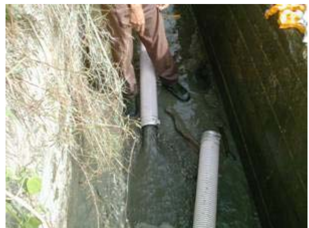
Flushing by siphon action at a head of 0.8 m
