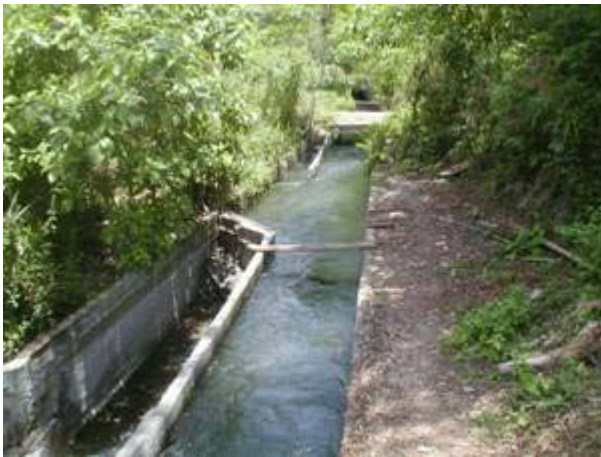
Side overflow spillway section, bow being Blocked with concrete to avoid leakage
