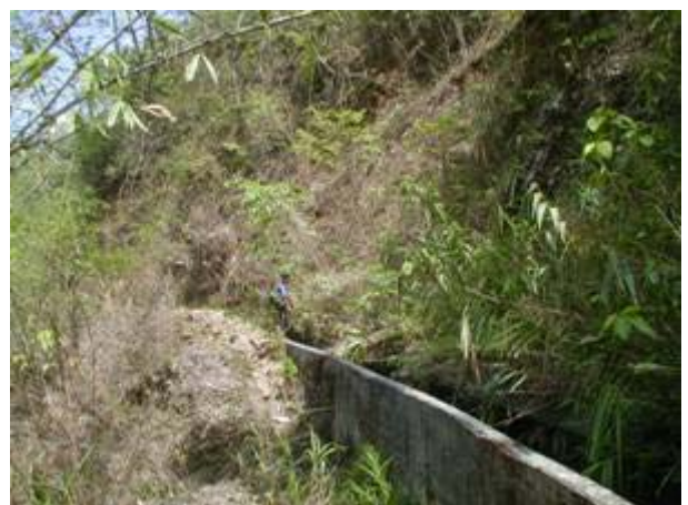
Debris once entered into and removed outside beside the channel. These channel sections should be placed with concrete cover.
