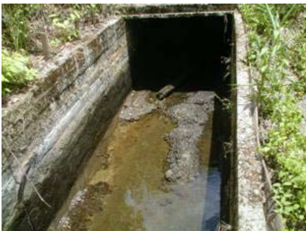
Erosion of channel floor
