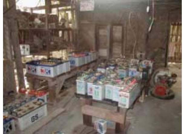
Many Batteries Charged in Serial Connection
