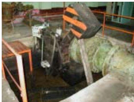
Inlet valve, locked at full open position
