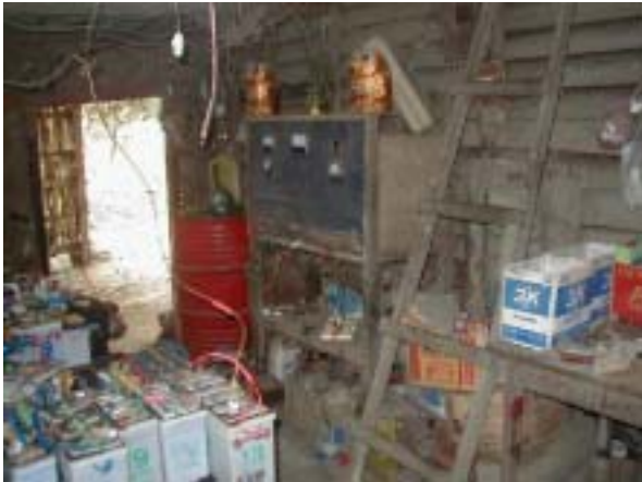
Typical BCS Powered by Diesel Generator
