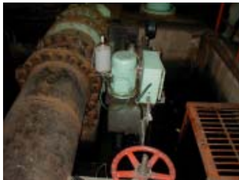
Hydraulic for valve operation
