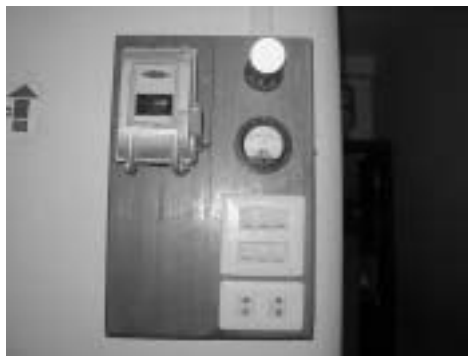
Receiving voltage at hotel at 200 V
