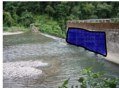
Skimmer wall at inlet
