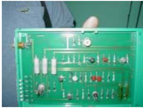
Damaged board of Thyristor controller
