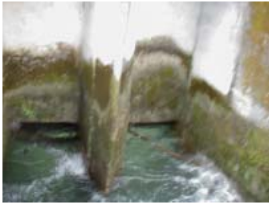
Flow at intake gate, trees clogged in the opening on the right side
