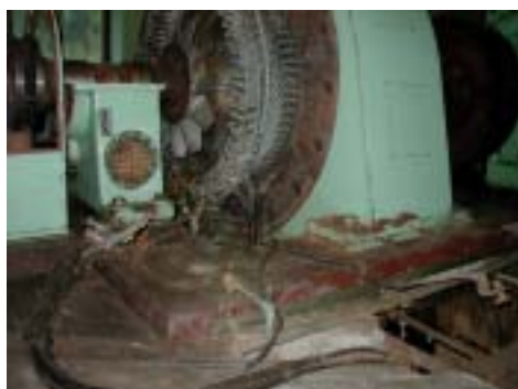
Cooling pipe that broke and watered stator coil
