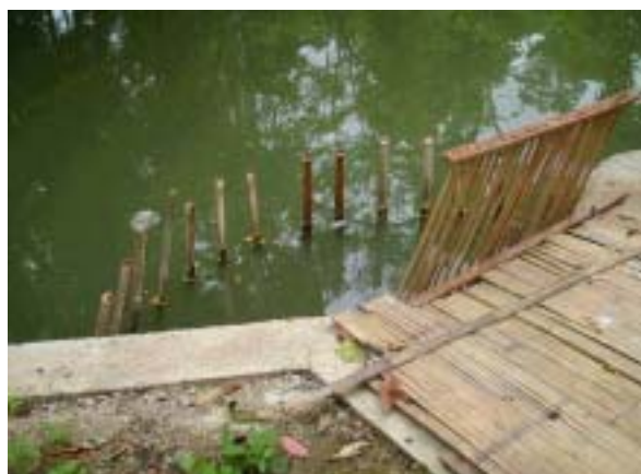
Sample of Intake Trashracks Primary racks for flowing trees combined with secondary racks for tree leaves.
