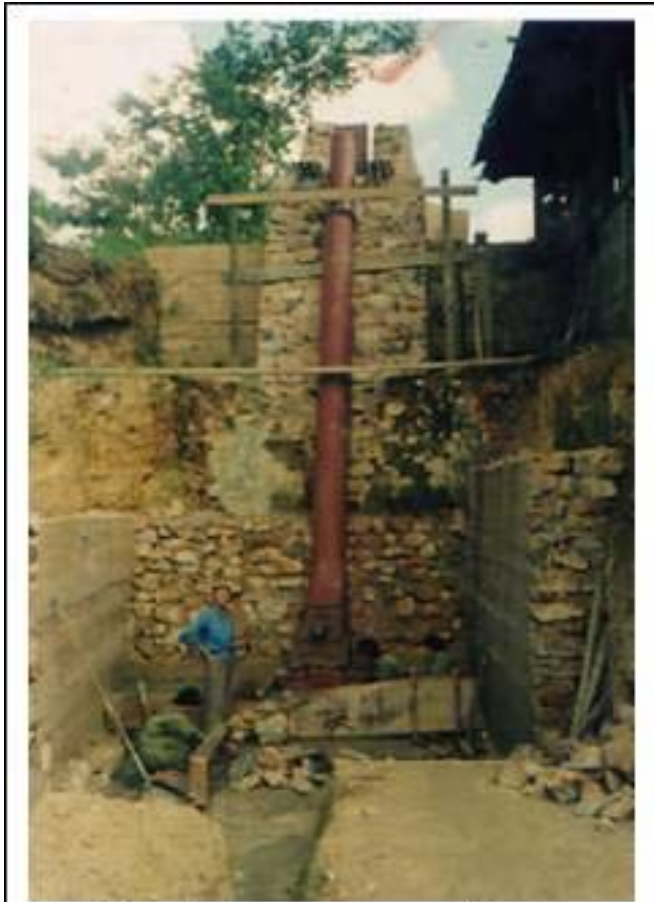
Penstock on Masonry Slopes Penstock is placed on stone masonry to a adjust to site topography. Mine Pon
