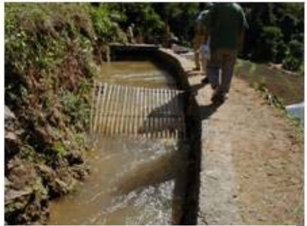
Head Tank with Trashracks
