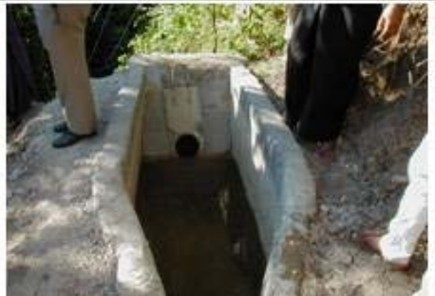
Head tank too small, no trashracks and floating debris can clog the penstock inlet
