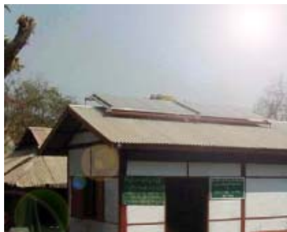
Solar Panel of BCS
