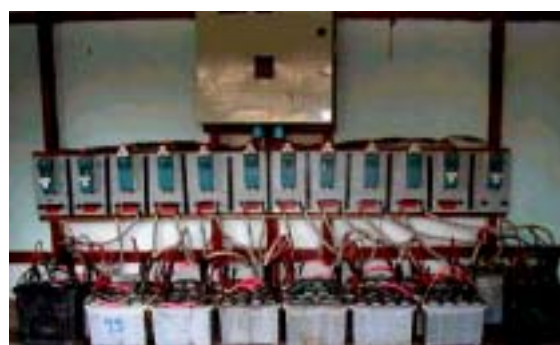
Battery charging at BCS
