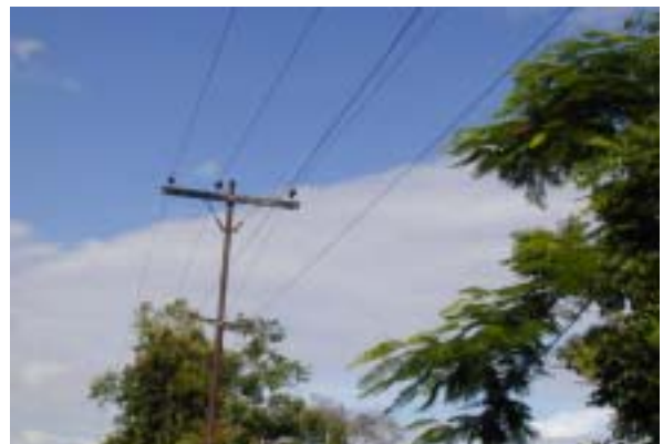
Distribution lines. Upper lines are of MEPE. Lower lines are installed by SPDC and transferred to MIC.
