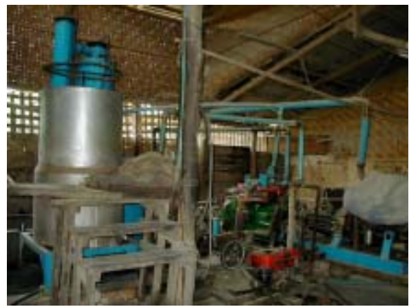
2. Generation System Beside Rice Mill
