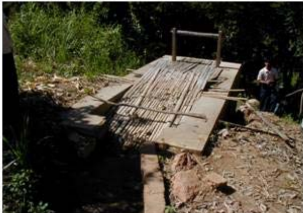
No spillway and side walls are not high enough to avoid water spilling
