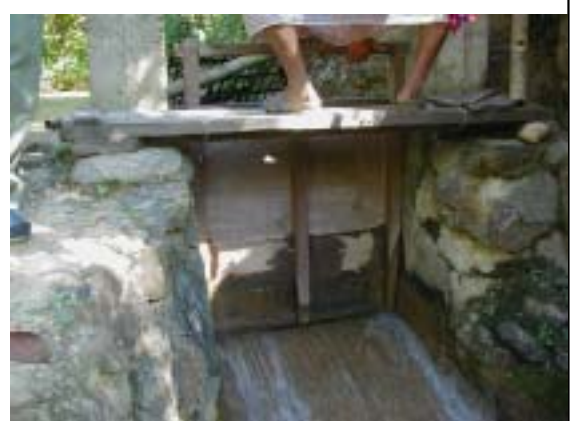
Wooden Hand-pull Gate Just start opening. The wooden gate well functions. Tha Le Oo.
