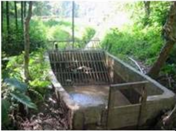
Head Tank and Bamboo Trashrack
