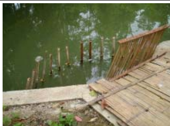
Sample of Intake Trashracks Primary racks for flowing trees combined with secondary racks for tree leaves.
