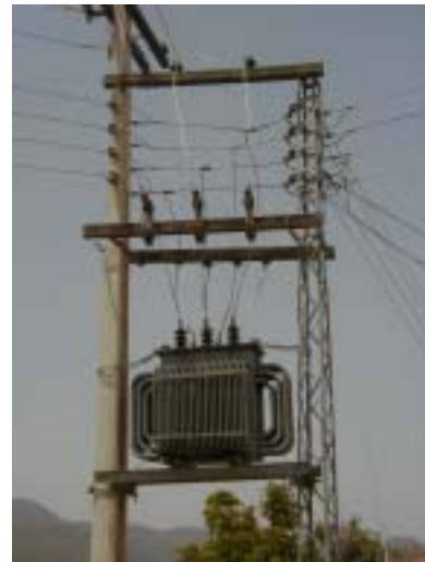
Transformer of this area
