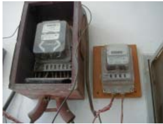
Power supply equipment
