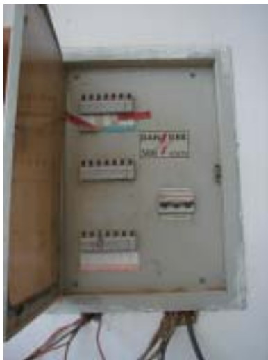
Power supply equipment
