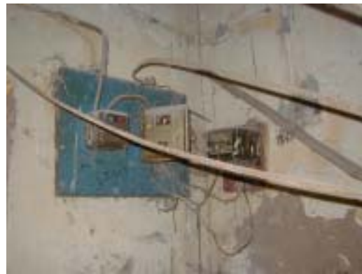
Power supply equipment and switch of the siren
