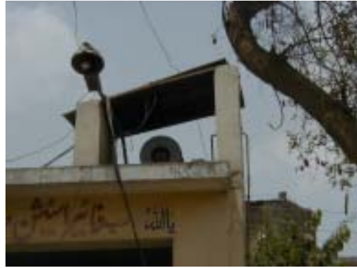
The siren installed on the roof
