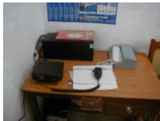
Transmission equipment for the transceiver
