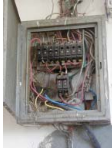
Power supply equipment
