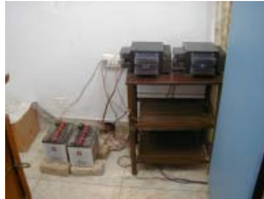
Battery and charger for the solar panel
