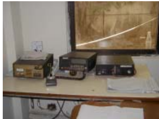
HF transmission equipment
