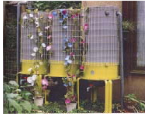
Storage Tank in House Lot
