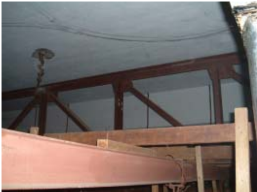
① Existing Steel truss Three steel trusses were installed behind ceiling for the purpose of support suspension loads.
