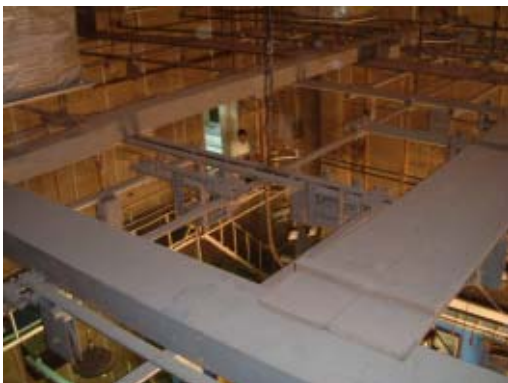
④ Piping grid and wiring rack
