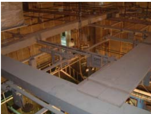
④ Piping grid and wiring rack
