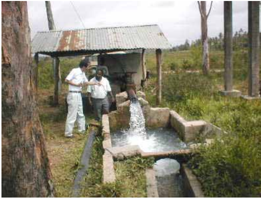
Active pump station
