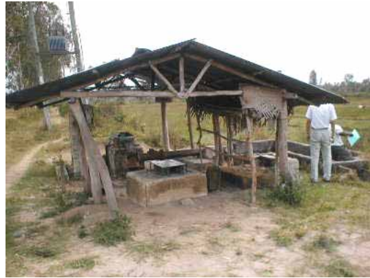
Damaged pump station
