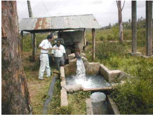
Active pump station
