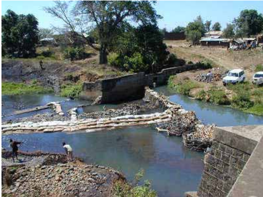
Collapsed intake weir
