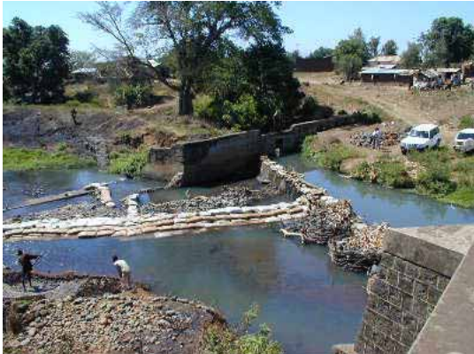
Collapsed intake weir
