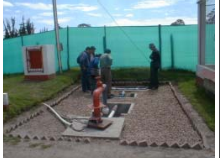
Pumping well for floriculture. Floriculture needs much groundwater. Therefore, conservation of groundwater is necessary.
