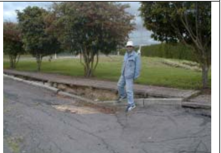
Depression of road in Siberia out of Bogotá City. Relation between depression and groundwater pumping was surveyed. However, there is no evidence between them so far.
