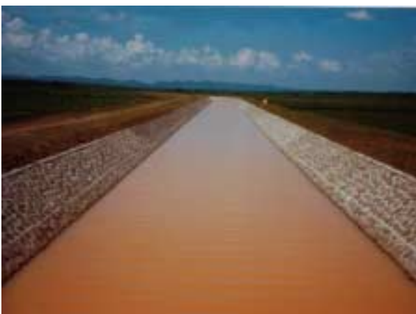
Figure-10 Lodoyo Irrigation Canal
