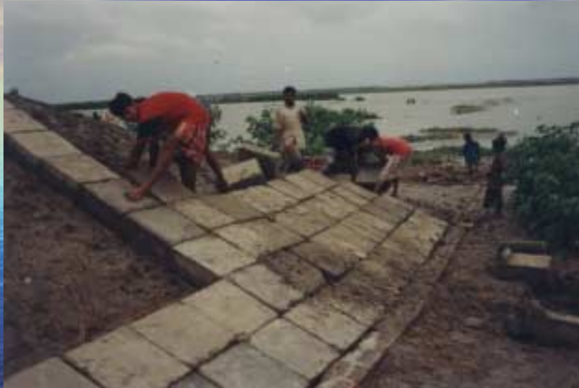
Slope Protection by CC Block in Haor Area
