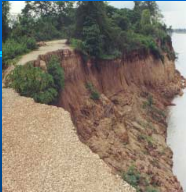
A road destroyed by riverbank erosion
