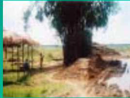
Construction of Mound Dike, Baquero Sur, Moncada, Tarlac under Package III (September 2002)
