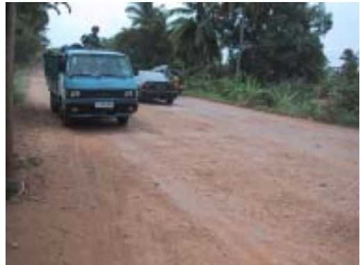
Destroyed pavement at Km 18~Km 19
