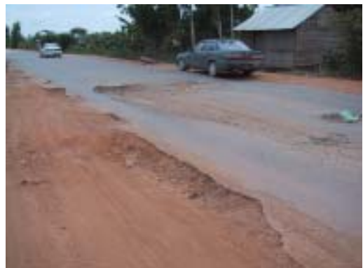
Another case of damaged pavement
