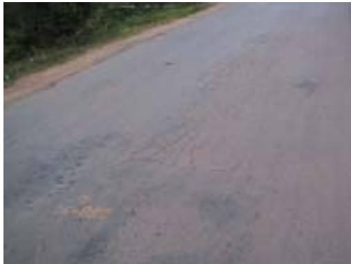
Crack are developing
