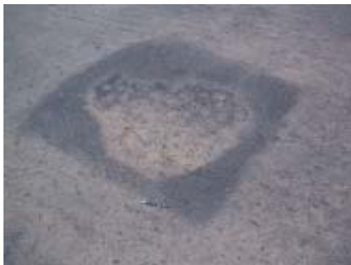
Previously repaired pothole
