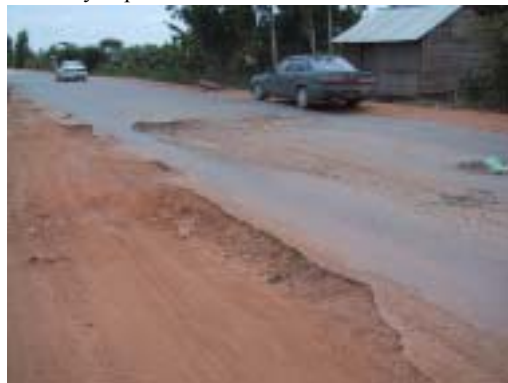
Another case of damaged pavement
