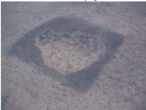
Previously repaired pothole
