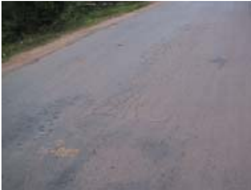
Crack are developing
