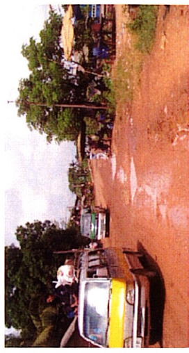
Deteriorated Pavement Condition
