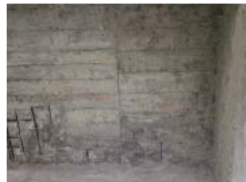
13. Km 50+040 Kampong Phnom Water Gate Scale, exposed re-bars and refilled concrete on the bottom surface of slab
