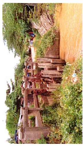
Deteriorated Old Colmatage Water Gate
