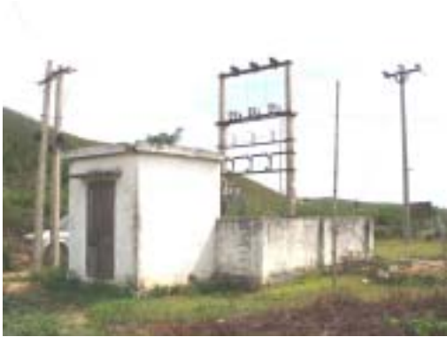
Existing Substation: T2NK1 M2
