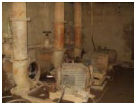
Pumps in Nam Trung Pumping Station
