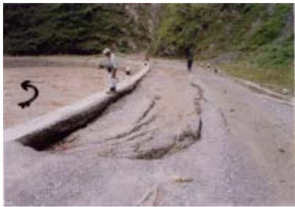
< Photo 2 > Type B-1: Scouring Crack and/or settlement on road surface
