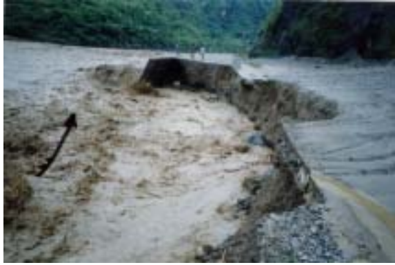
< Photo 5 > Type B-4: Scouring Washing away of embankment
