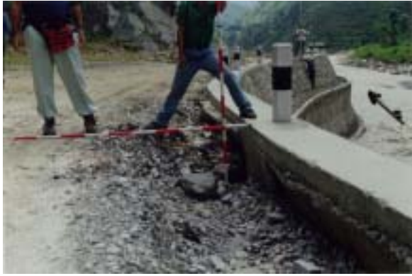
< Photo 1 > Type A: Erosion of road surface by surface water
