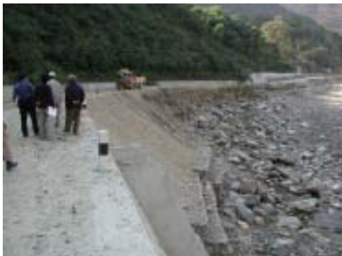
[No.44] STA.14+885 - 14+925 : Erosion of riverbank ( Temporary work was done by DOR )
