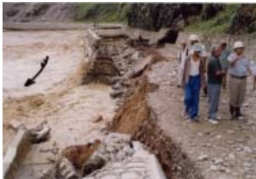
[No.65] STA.21+015 - 21+056 : Embankment washed away
