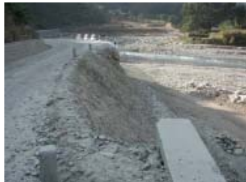
[No.50] STA.18+558 - 18+581 : Embankment washed away ( Temporary work was done by DOR )
