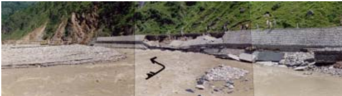
[No.18] STA.06+065 - 06+206 : Embankment washed away
