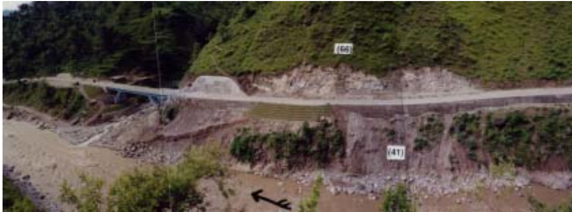
[No.41] STA.13+262 : Slope failure due to scouring
