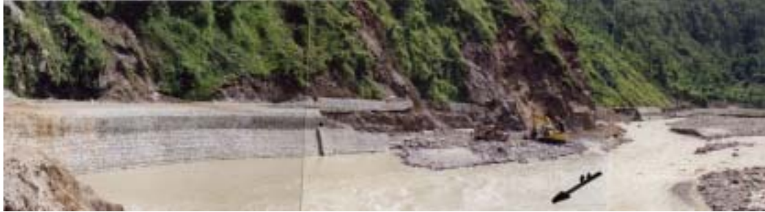
[No.17] STA.05+500 - 05+560 : Overturning of revetment
