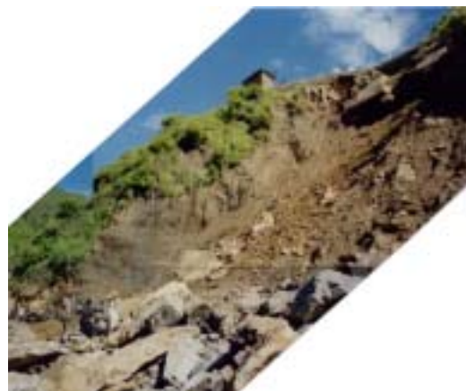
[No.66] STA.22+915 : Slope failure due to scouring
